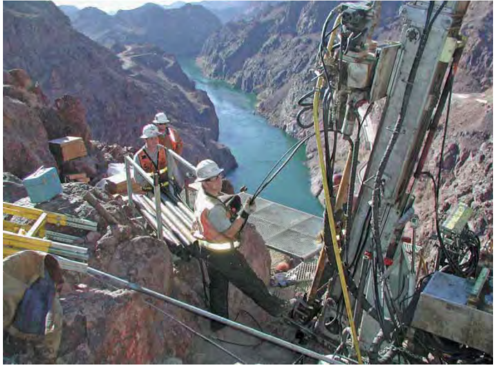
The Crux crews are using a Goodman Jack attached to a drill rod to test the strength of the rock at the Arizona abutment site.
