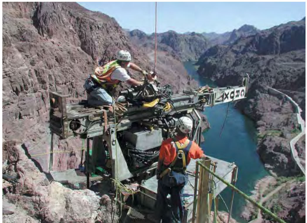
Drill rig being assembled with the aid of a helicopter at Nevada Skewback.
