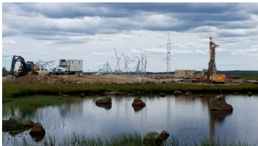
Figure 7. Boggy/wet ground conditions
