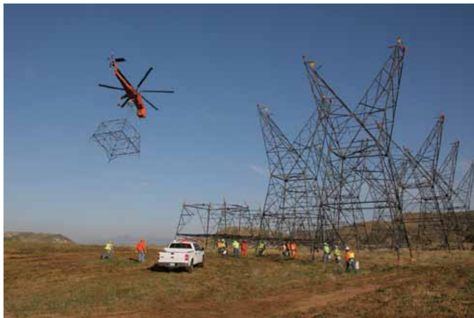
A sky crane flies out with a body extension for tower erection.
