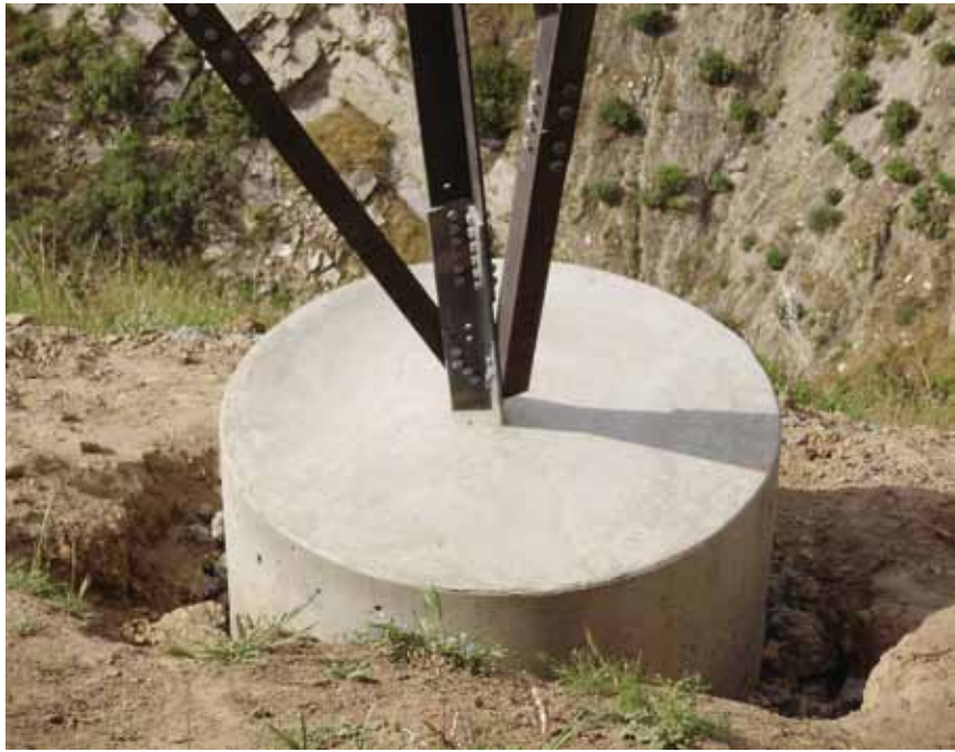
The final appearance of a micropile foundation does not indicate its internal structure.
