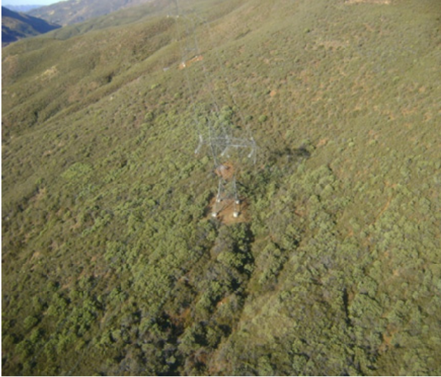
Figure 3: Micropile construction with helicopter support minimizes the disturbance footprint required for foundation construction. Typical actual vegetation clearing is less than 50 percent of the SUP approved disturbance.
