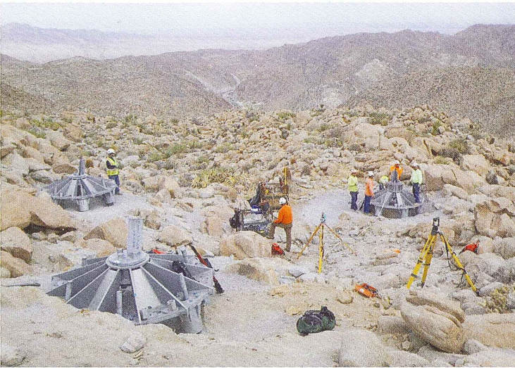
Surveyors set final stub angles to ensure proper batter and distance for tower erection in Mountain Springs Grade.
