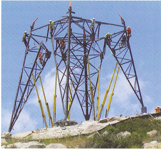
With the assistance of the yellow leg brace kickstands, a PAR crew ties four tower legs together.
