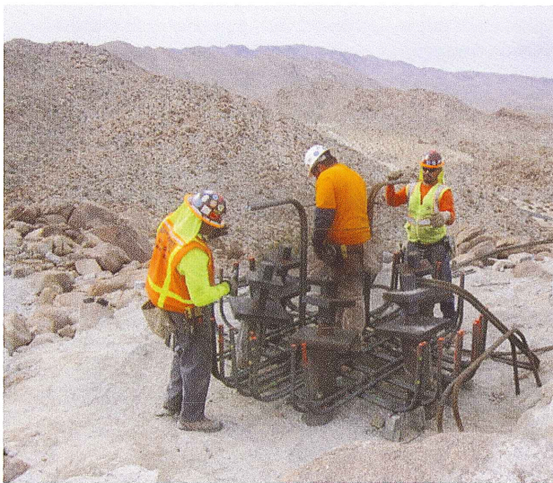
Pile cap constructors tie reinforcing bar for concrete placement in Mountain Springs Grade, Imperial County, California.
