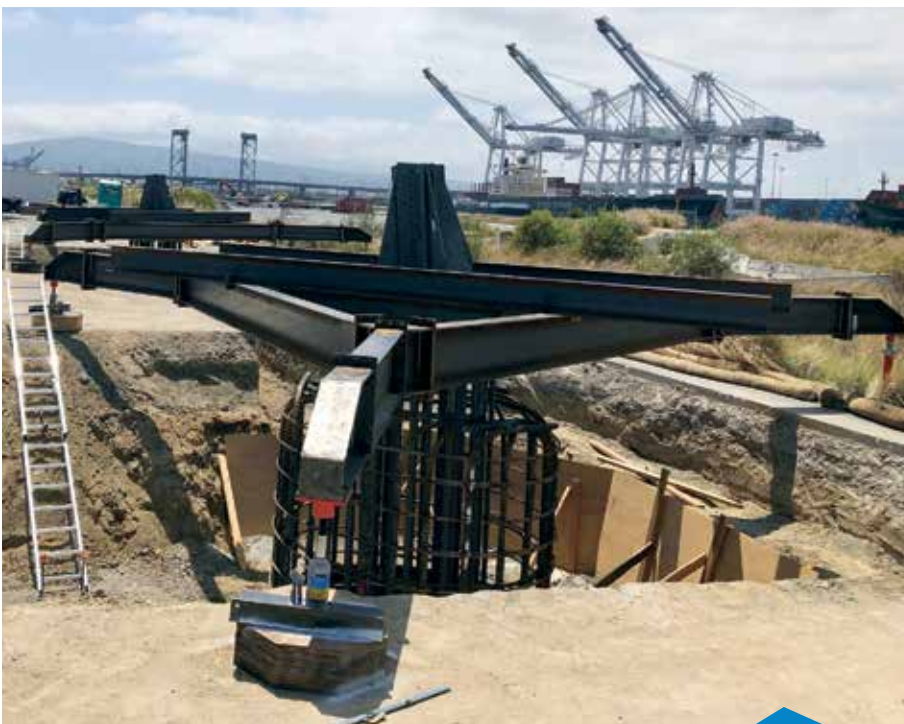
STUB ANGLE AND HEAVY SUPPORTS
